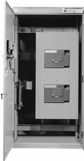
3000 Amperes, 4-Pole, NEMA 1 Enclosed
